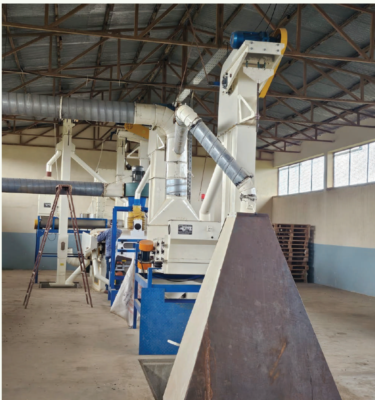
Figure 15: Installed seed cleaning and processing machine at Adi-Zarna for use by NARI and AED, Eritrea
